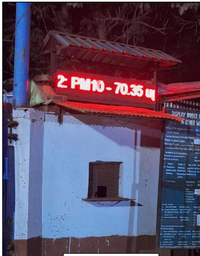
CAAQM installed in unit
