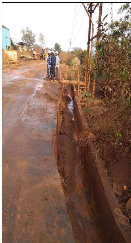
Spillage collection channel inside unit
